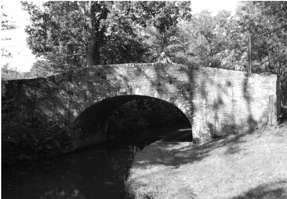
Plate 1. Going nowhere – Bridge 123. 'Spiteful Lane' Bridge in 1857 but today seemingly misnamed as 'Pen-y-bryn' Bridge. It now offers no road or field access (although does provide access to the towpath).
