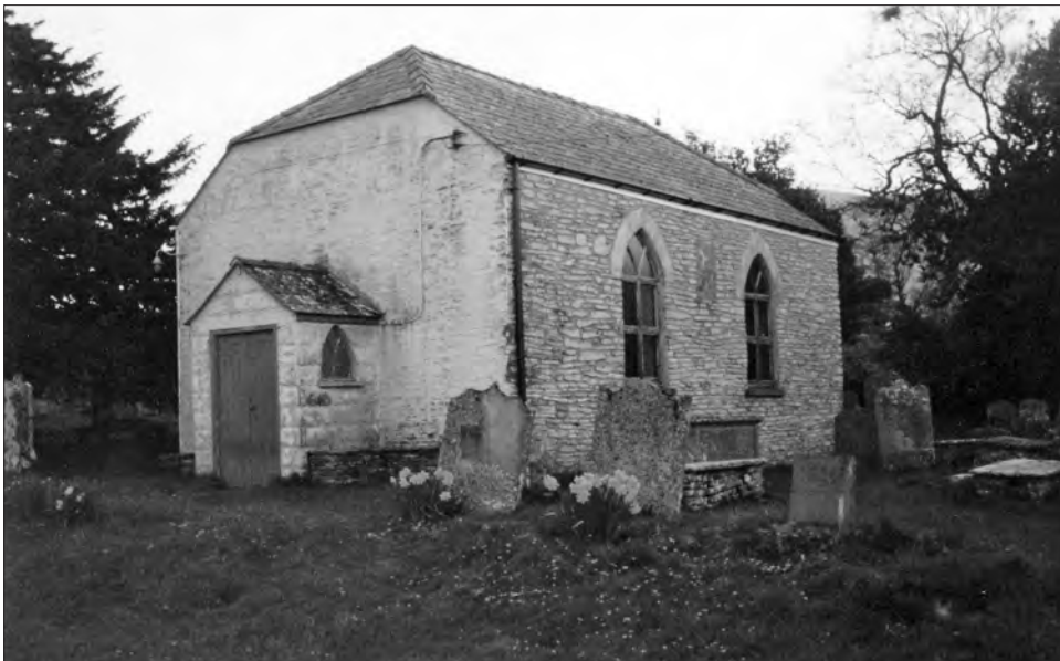
Figure 3 Penyrheol Chapel c.2001. Front and side elevations viewed from the north-west. The plaque between the two windows commemorates the gift of money from Thomas Williams of The Island, c.1788.
